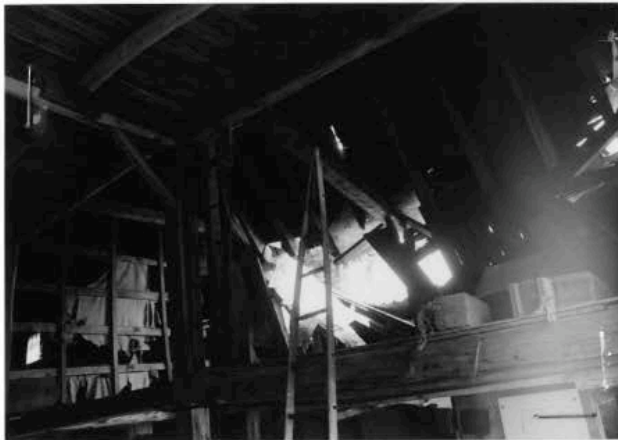
Barn-interior - failed roof. 5/01.
